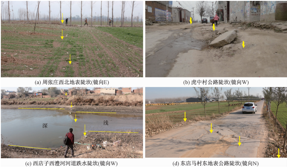
图 4 隆尧地裂缝地表陡坎 Fig.4 Surface scarcity of the Longyao ground fissures
