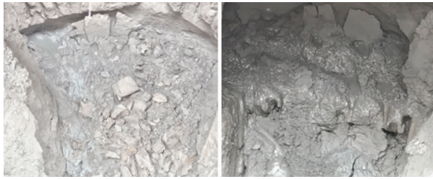
图1 武汉万象城基坑厚互层土中“流砂”和“流水”现象 Fig.1 Phenomenon of “quicksand” and “flowing water” of thick interbedded soil in Wuhan Huarun Wanxiang
