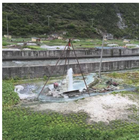
图1 川藏铁路沿线典型钻孔自流现象 Fig. 1 Typical artesian borehole along the Sichuan-Tibet Railway
