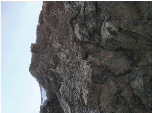
图 7 老虎嘴路段凹岩腔卸荷裂隙图 Fig. 7 Picture of fissures in concave rock cavities of Laohuzui road section after the earthquake
