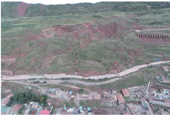
图 5 前缘鼓胀引起房屋倒塌 Fig. 5 The swelling of the front edge caused the houses to collapse
