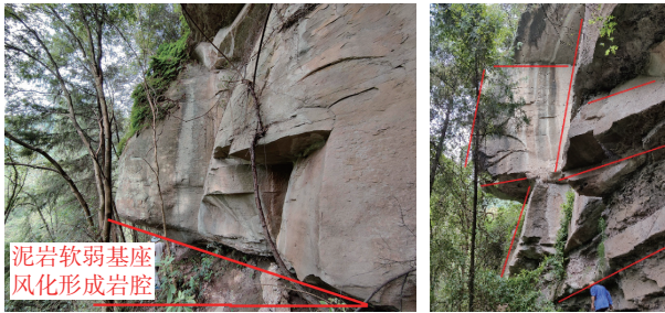
图 4 泥岩软弱基座和节理切割 Fig. 4 Mudstone weak base and joints cutting
