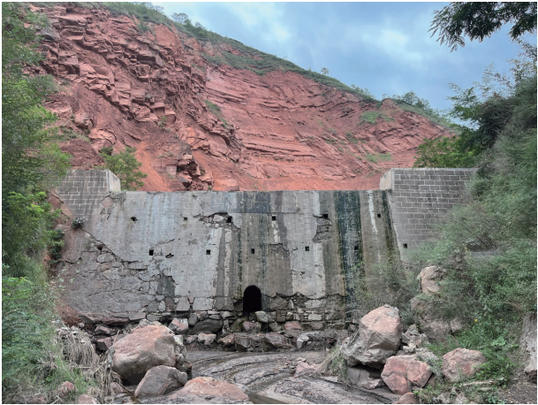
图 5 马槽沟 12 号坝现状 Fig. 5 Current state of dam No. 12 in Macao gully
