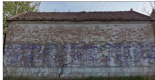
图 6 龙东煤矿近年开采造成建筑开裂 Fig.6 Construction cracking caused by recent mining in Longdong coal mine
