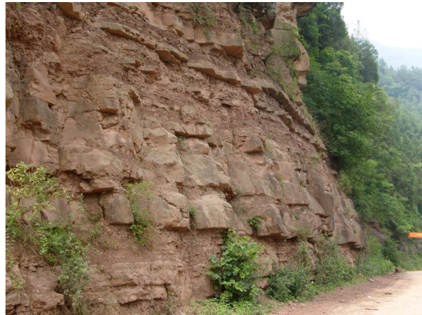
图9 雷神庙崩塌(危岩)危及公路 Fig.9 Rocks of the Leishen temple that endanger road
