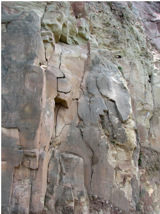
图2 砂岩内发育的不规则、陡倾卸荷裂隙 Fig.2 Irregular fractures developed in the sandstone
