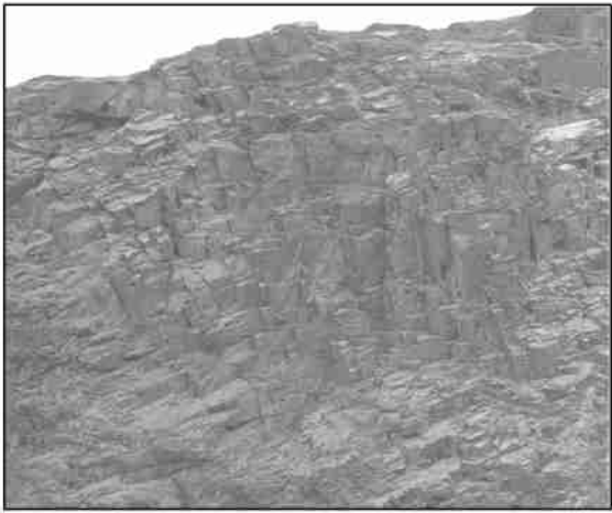
图2 斜坡岩体破碎 Fig.2 Cracked rock of slope
