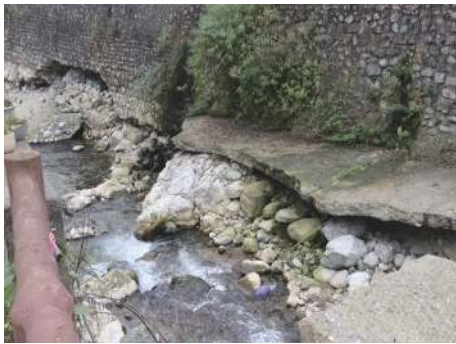
图 6 侧墙被块石破坏严重 Fig. 6 The side wall was seriously damaged by the block stone
