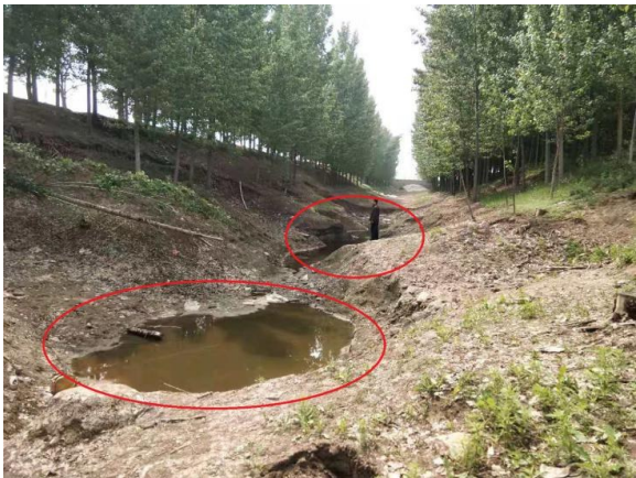
图6 土山村串珠状岩溶塌陷 Fig. 6 Cluster karst collapse in Tushan village
