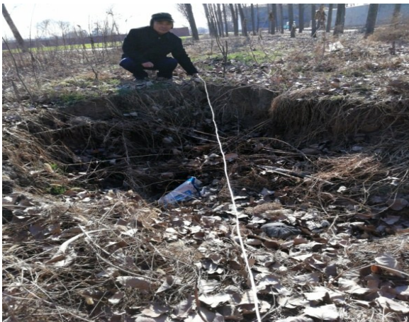
图7 尹家庄地势低洼处岩溶塌陷 Fig. 7 Karst collapse at low-lying places of Yinjiazhuang village
